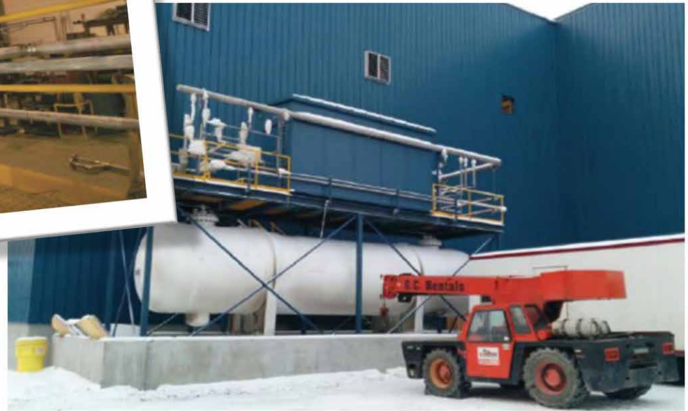
Liquid SO 2 Storage Tank & Tank Housing
