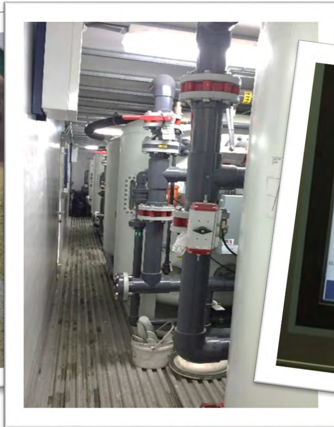
Automated IX Pilot Trailer Fitted with 6 IX Columns
