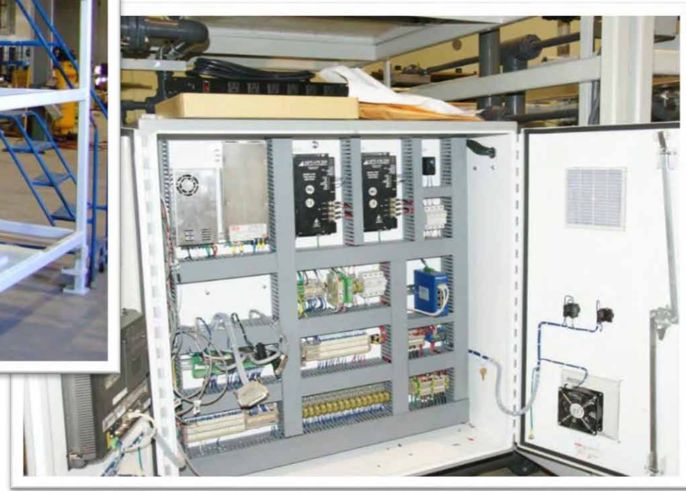
VRP Pilot – electrical & controls panel
